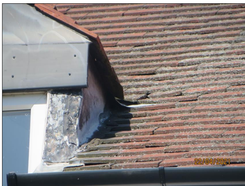
Figure 14. Lead flashing raised around upper floor window on rear elevation.
