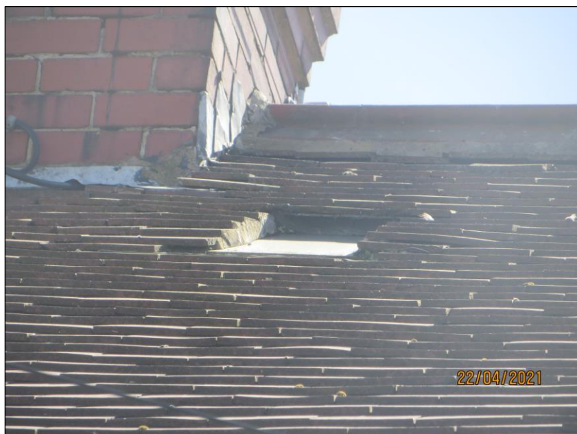
Figure 11. Gaps present around misaligned/slipped tiles on front elevation.
