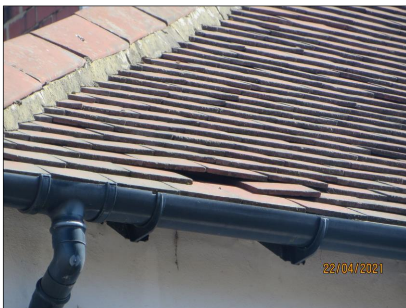
Figure 12. Gable end, with a missing tile lower down.
