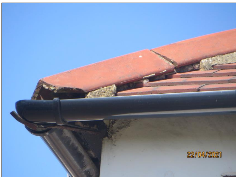
Figure 10. Gaps present along ridge tiles on the rear elevation.
