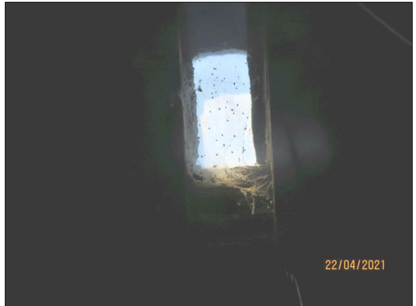
Figure 16. Cobwebs present within loft voids, particularly around the small window.
